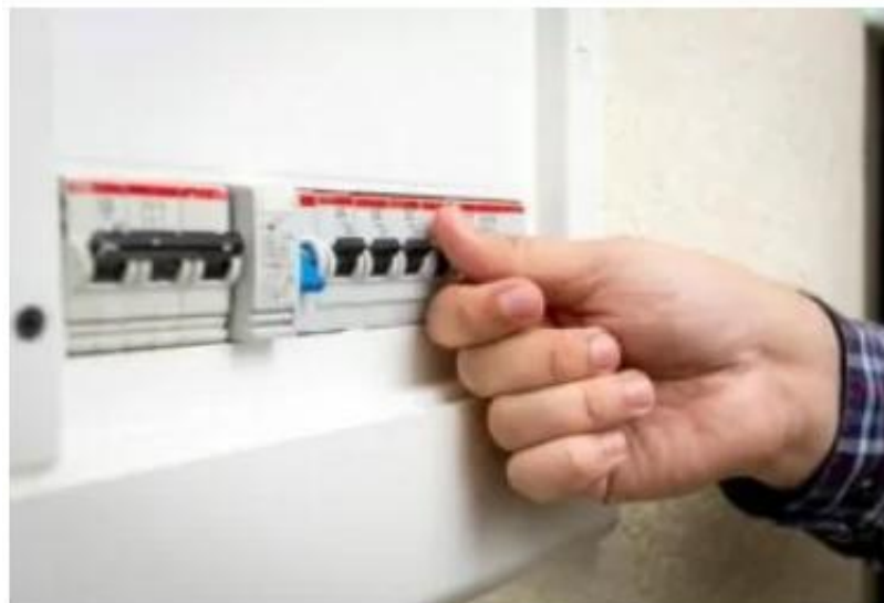
Figure 2. 1. Making Circuit Breaker Off
